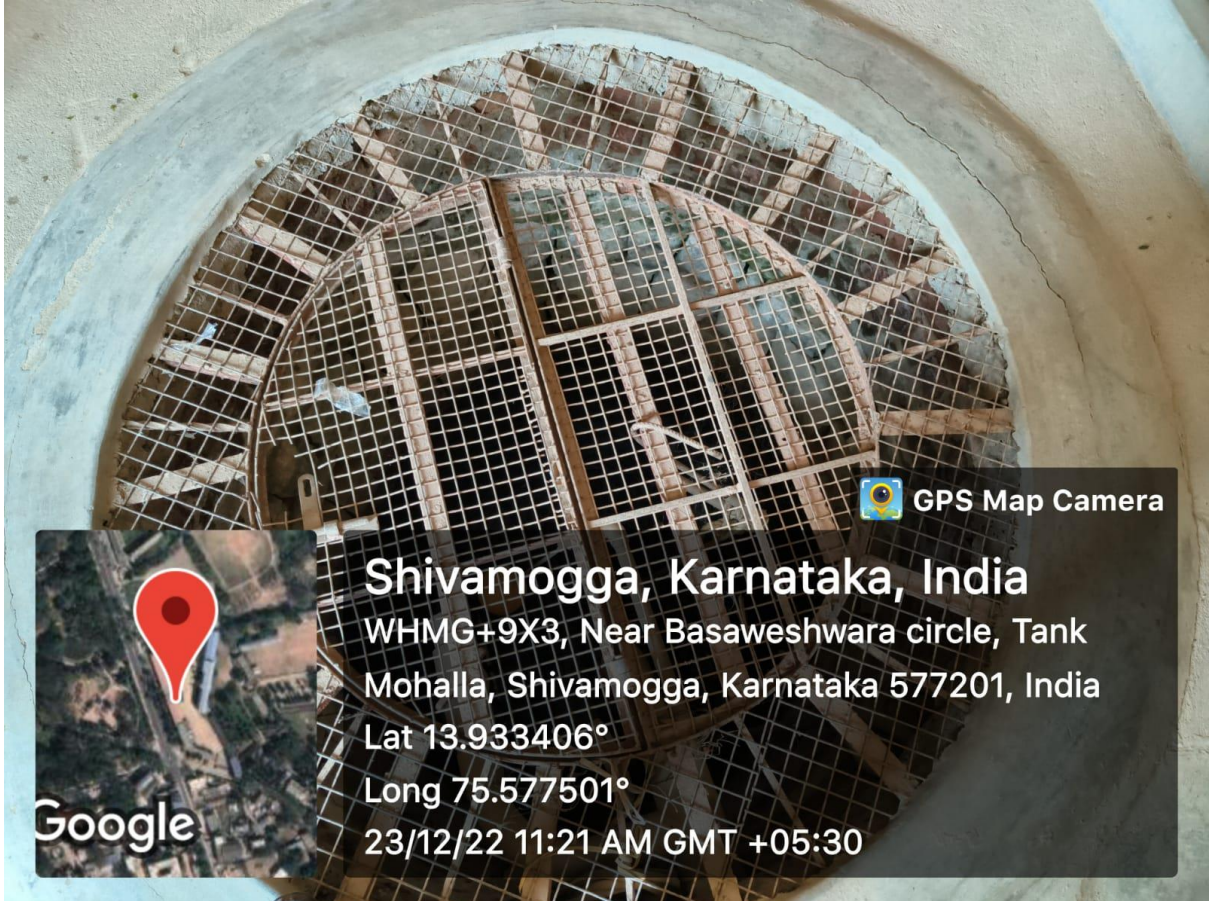
Open well recharge
