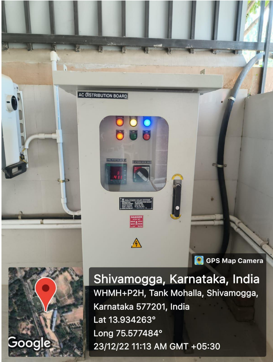
Solar Panels AC Distribution board installed in College Canteen Basement
