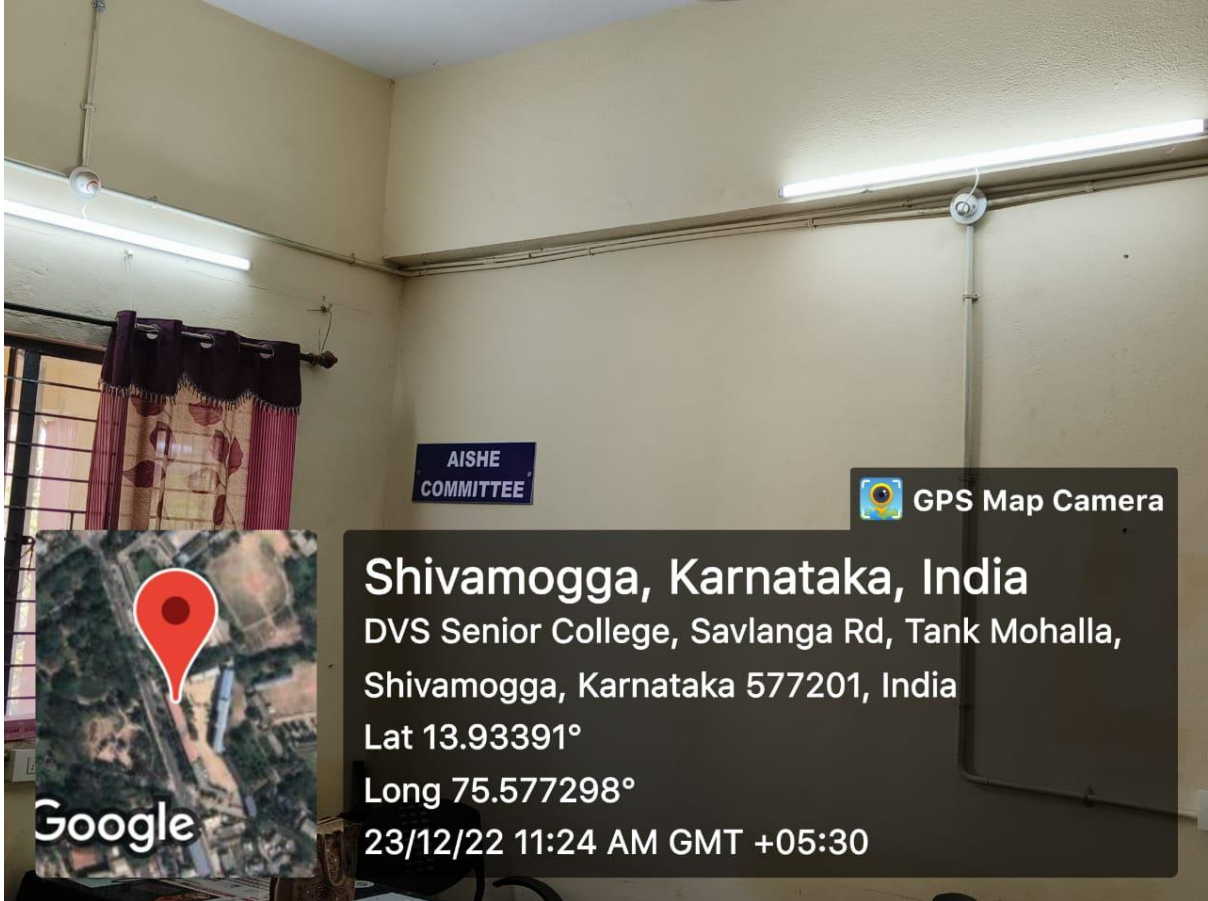
LED Bulbs used in chemistry staff room
