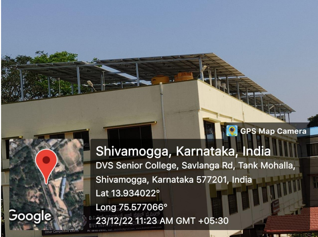
Solar Panels installed on the top of Management Building
