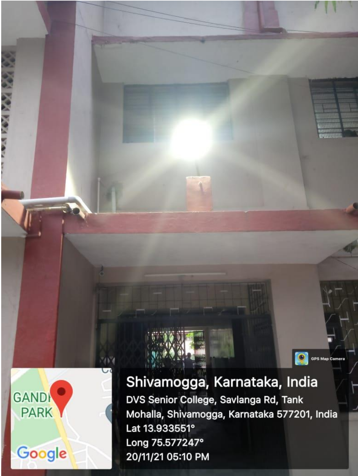
LED Bulbs in Entrance
