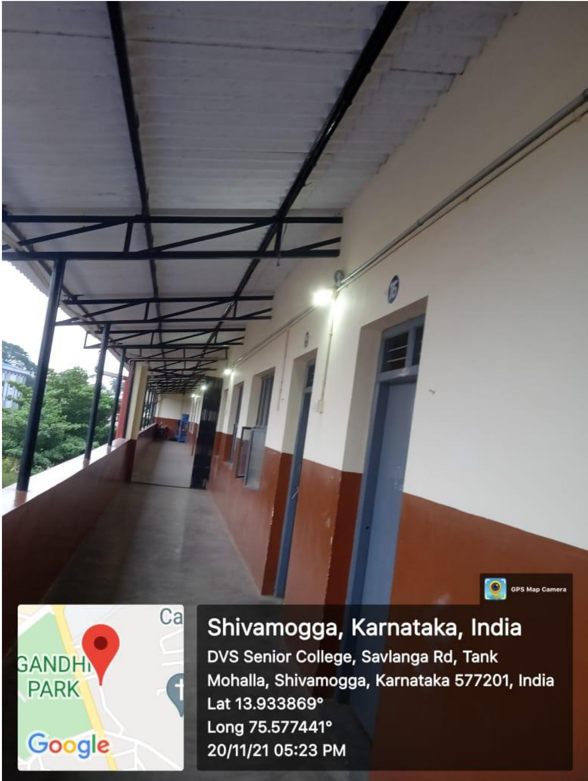
LED Bulbs in Corridor
